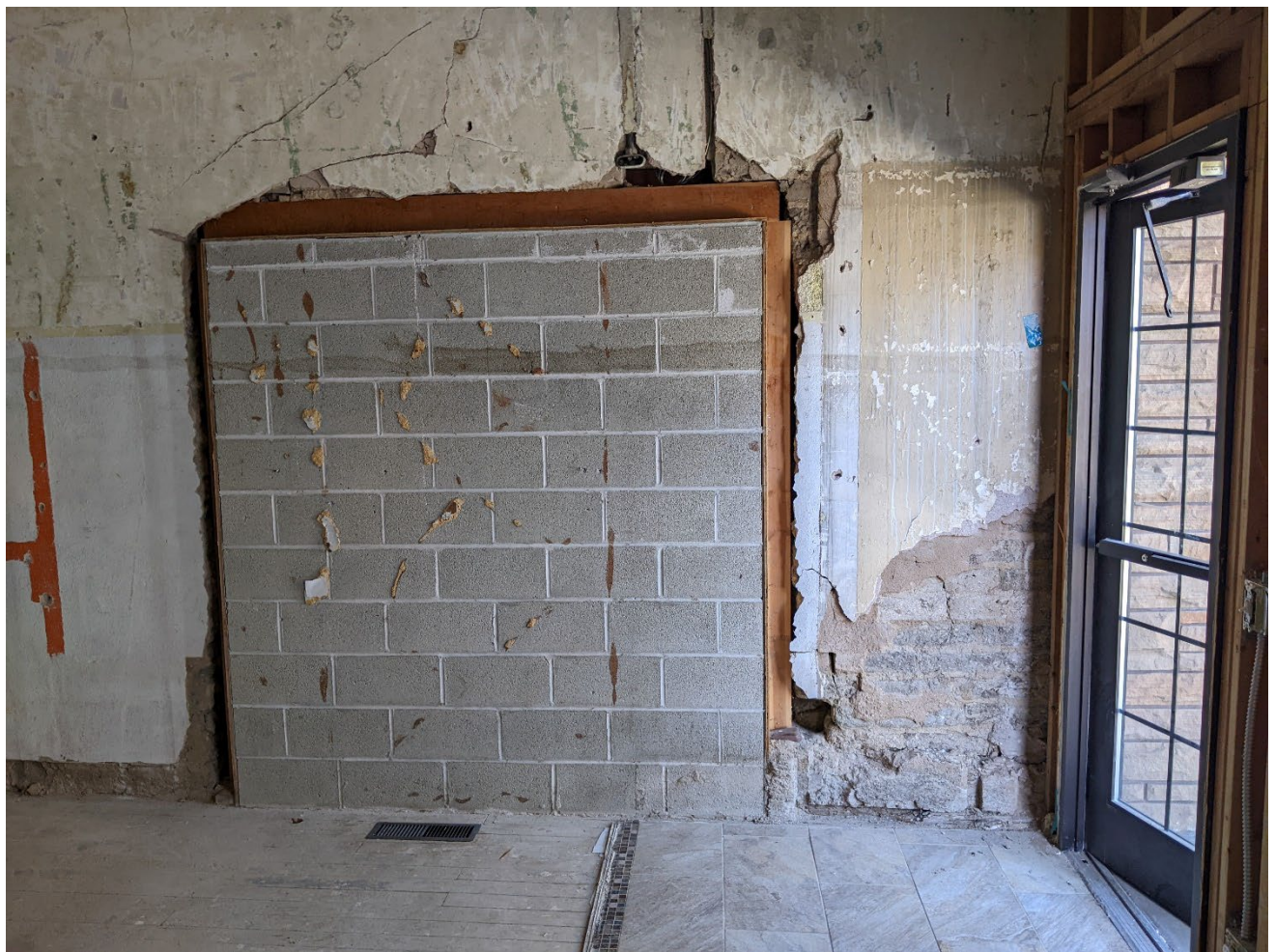
Patch and infill at Cappriotti's wall. Large holes and damage to the walls are also visible.
