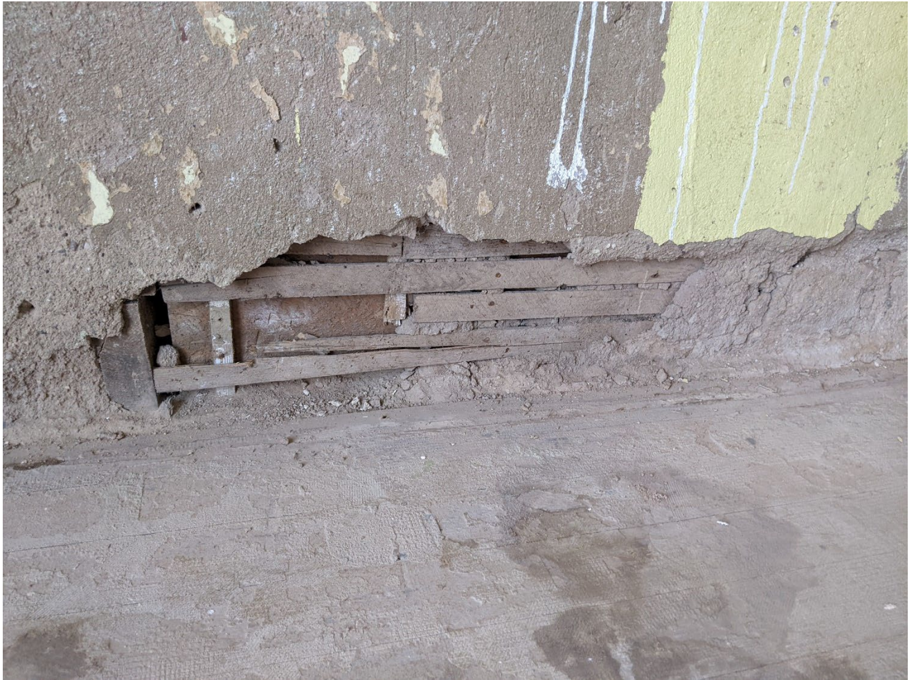
Deteriorating adobe wall at base. Large portions of plaster are missing from several areas and pose a safety risk when they fall from the walls.
