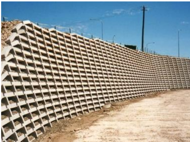
Figure 14.33A.2. Terracing and Retaining Wall – Not Permitted
