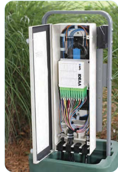
IDEAA Splitter Module and Exterior Distribution Enclosure in Pedestal
