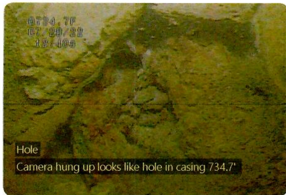
Hole | Camera hung up looks like hole in casing 734.7'
