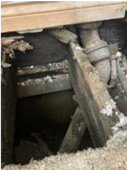
Subfloor condition at northeast corner.
