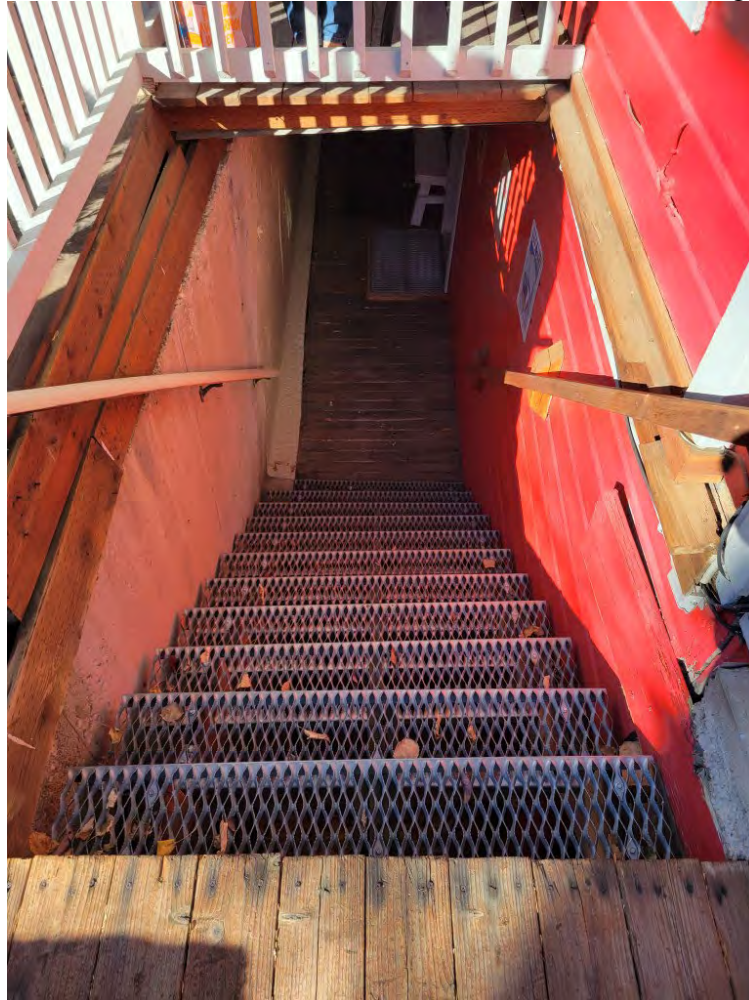
10 of 25. Stairwell access to lower level front entrance hall . Camera facing north and down.
