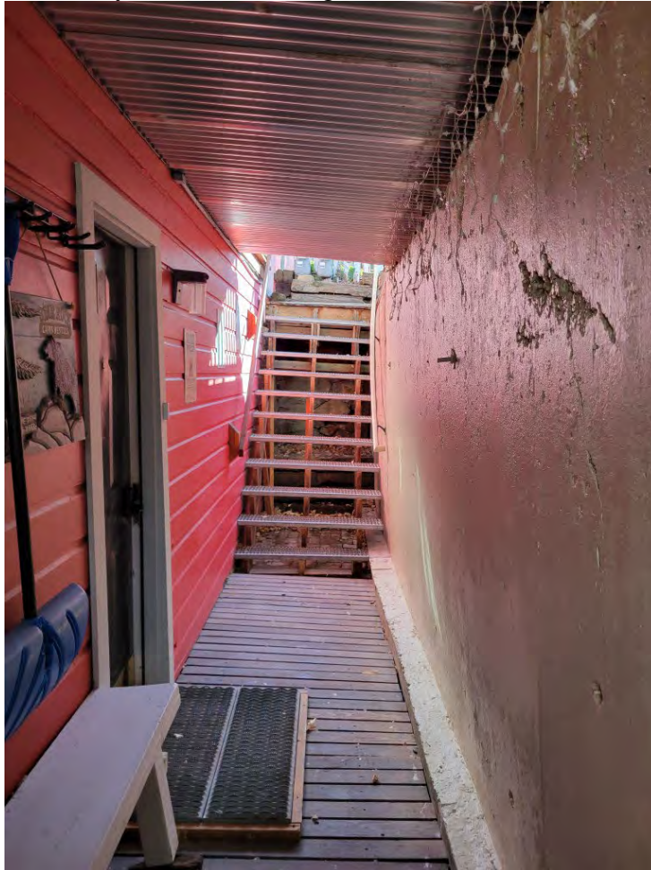
11 of 25. Front exterior entry hall and retaining wall, lower level. Camera facing south.
