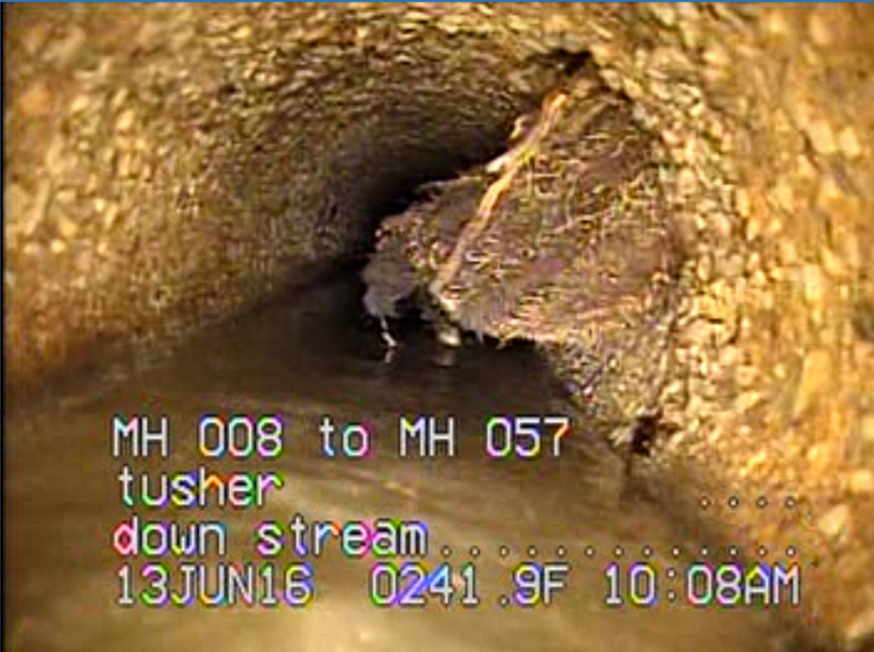
Roots in main under Tusher Street
