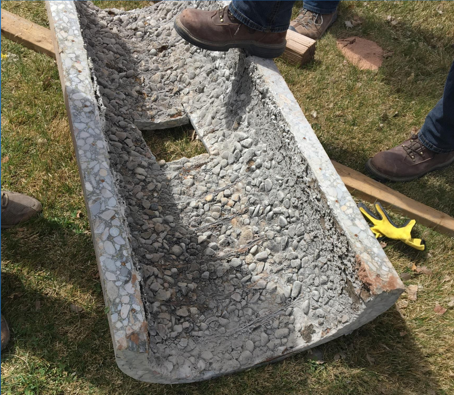
WWTP outfall pipe
