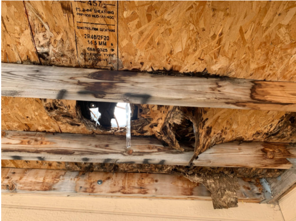
Image 11: Major roof damage in East Carbon Home
