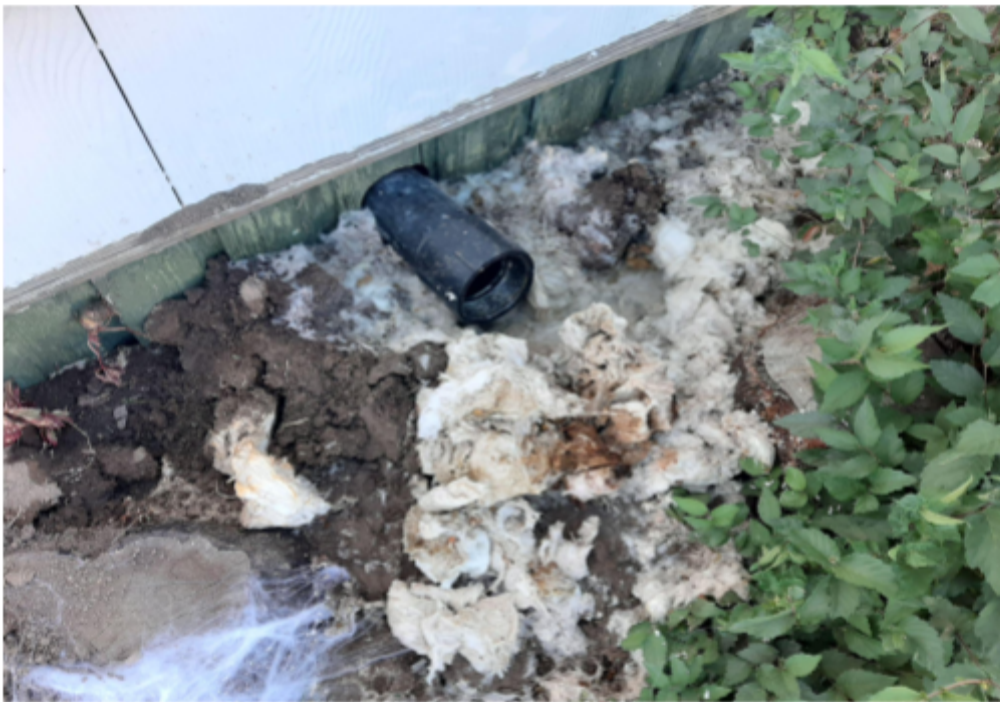
Image 9: Top, Sewer and Gray water backing up into a child's bathtub. Bottom, same home as top image, Wastewater backing up out of a clean out into front yard of East Carbon Home.
