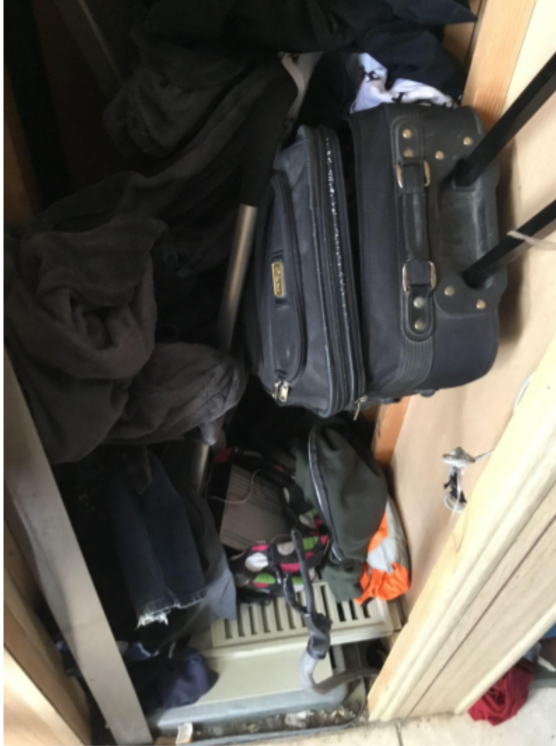
Image 2: Lack of furnace coupled with dangerous wiring practice in Melody Estates Mobile home park. Example of High density housing issue.
