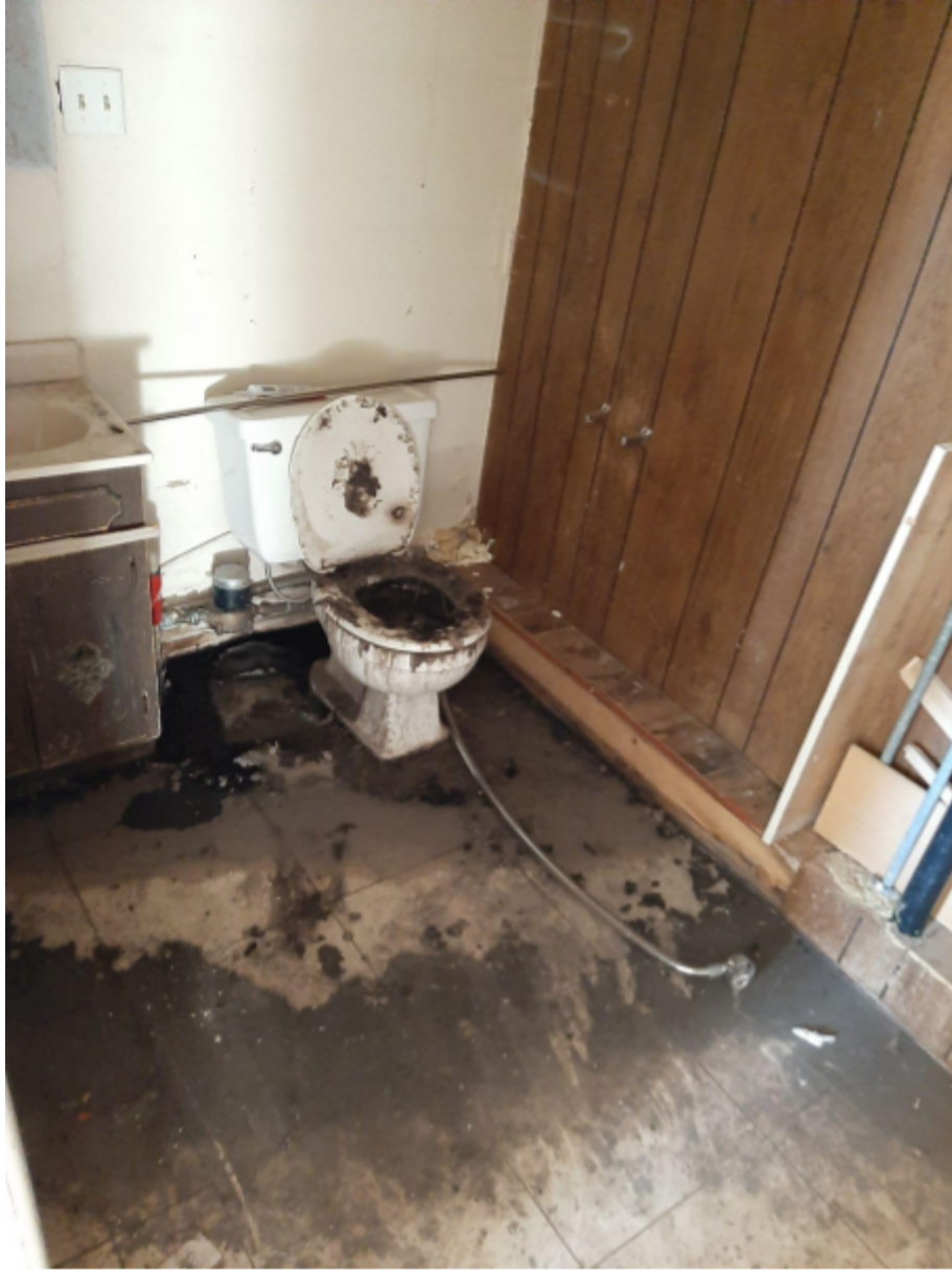
Image 8: Sewer backup in carbonville mobile home park.
