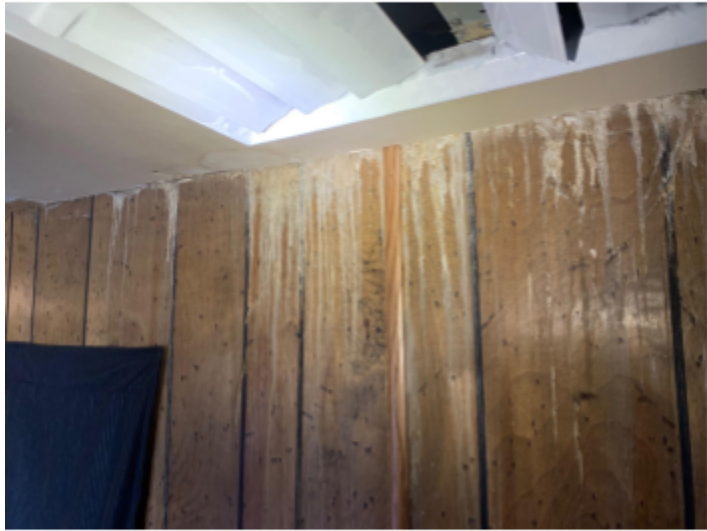
Image 1: Roof physically separating from trailer, associated severe water damage throughout trailer in Ferron. Example of low density housing issue.
