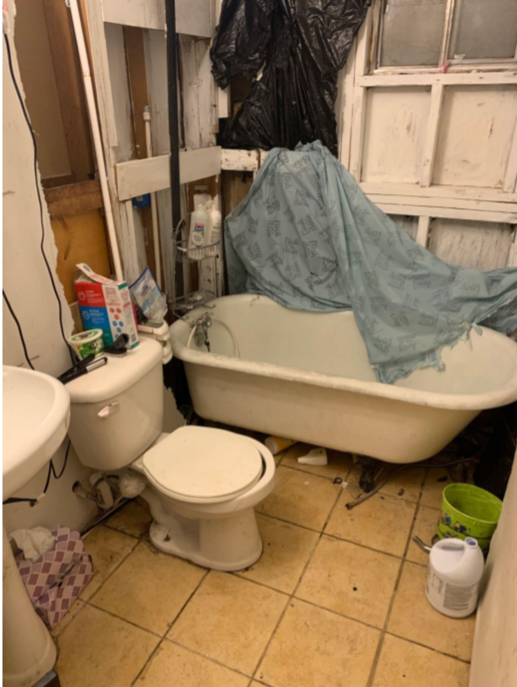
Image 6: Bathroom with no shower wall in East Carbon home.
