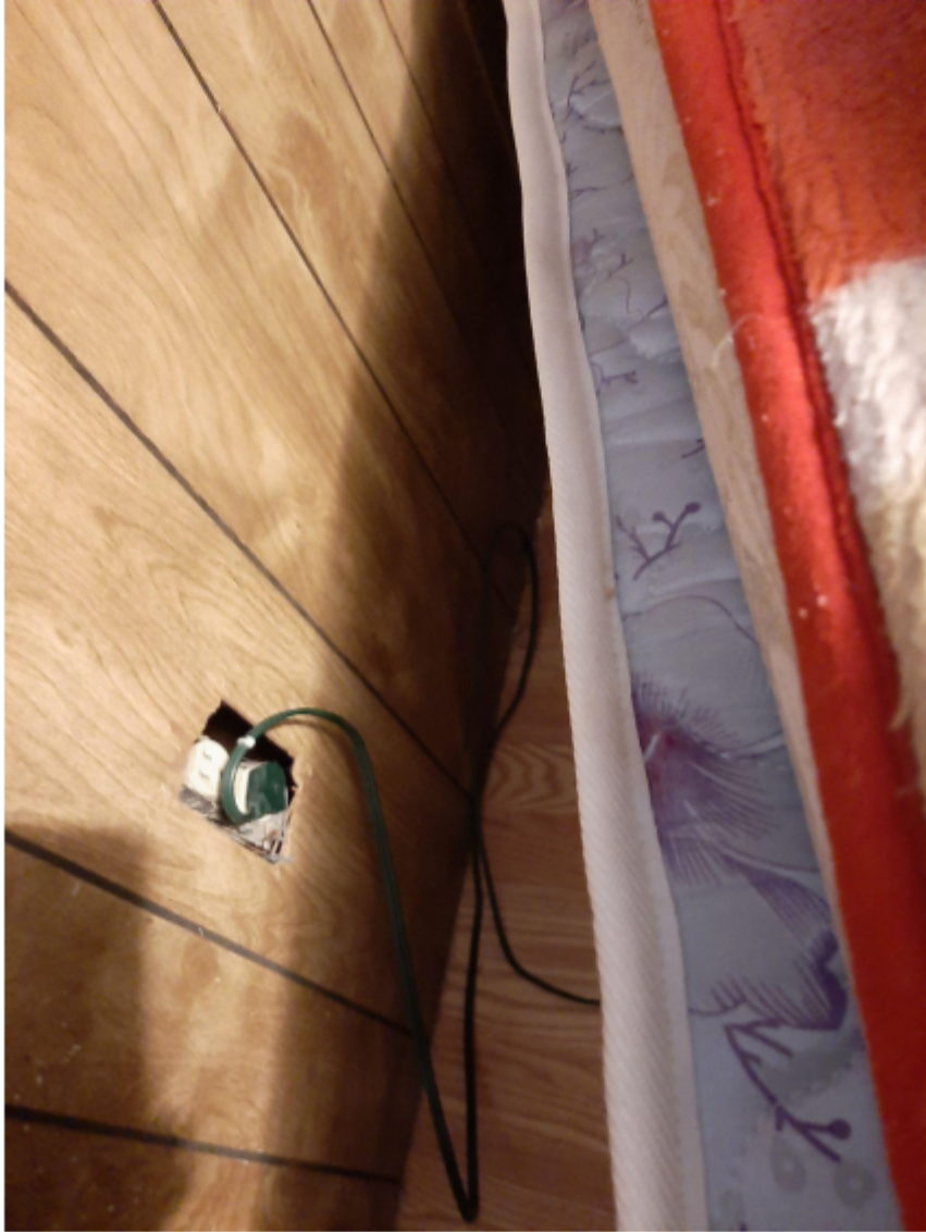
Image 7: unprotected and recessed electrical socket in child's bedroom in Price home.
