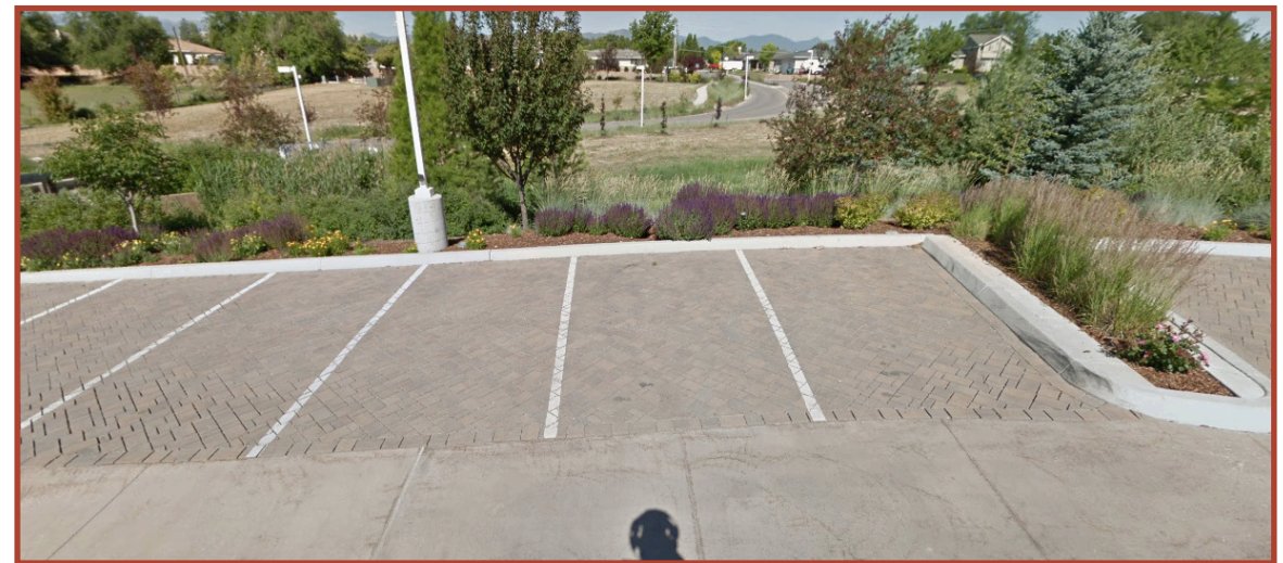
Pervious Pavers in Parking Stalls
