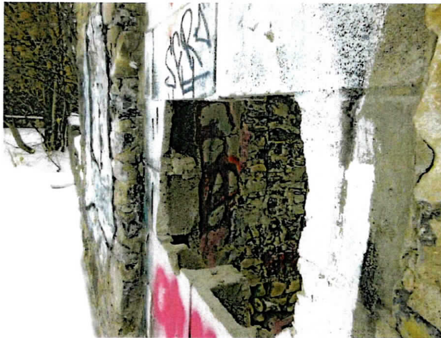
Photo 2 Damaged CMU masonry infill
