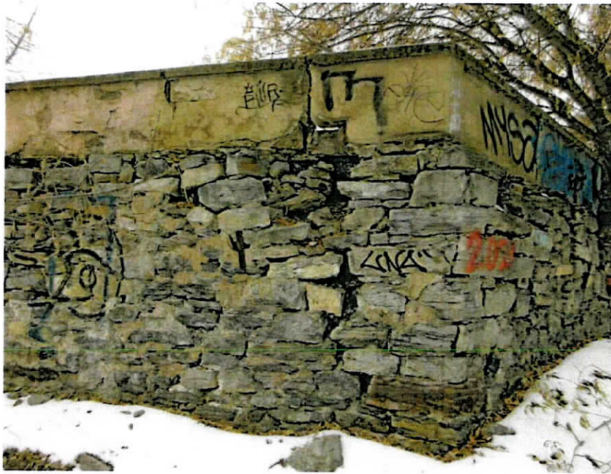
Photo 5 Missing mortar and crack in wall due to possible settlement
