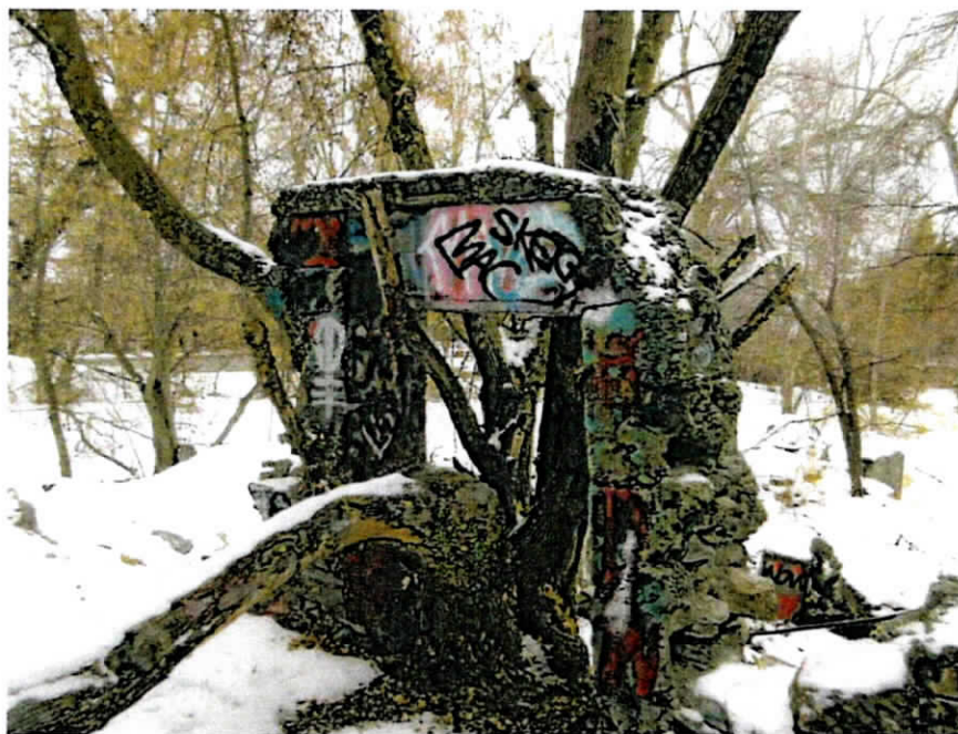
Photo 12 Tree growing through masonry wall
