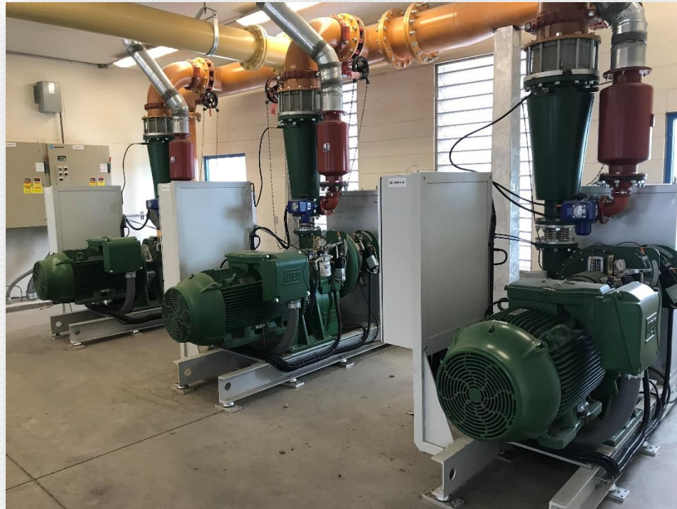
Aeration Blowers (6 total)
