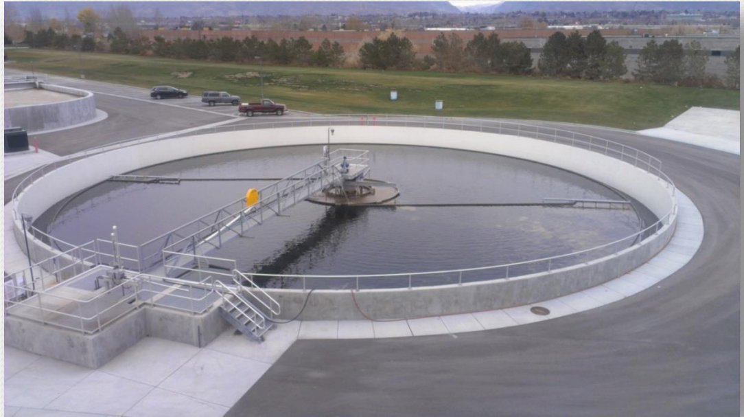
Secondary Clarifiers (4 total)
