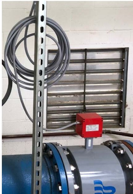
Flow Meter at Drinking Well #3
