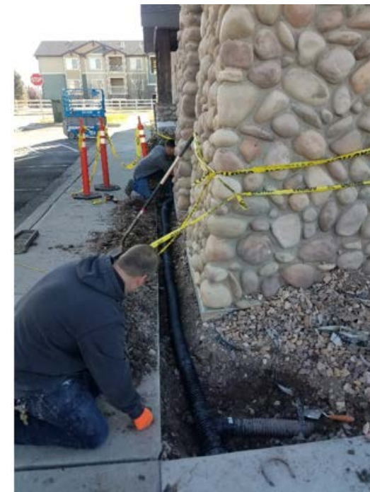
City Hall Downspouts
