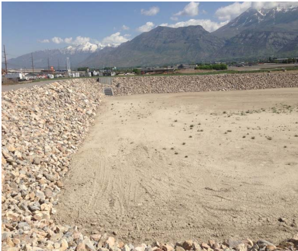
Williams Farm Detention Pond
