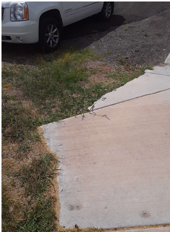
Figure 5. Damage Handicap Ramp
