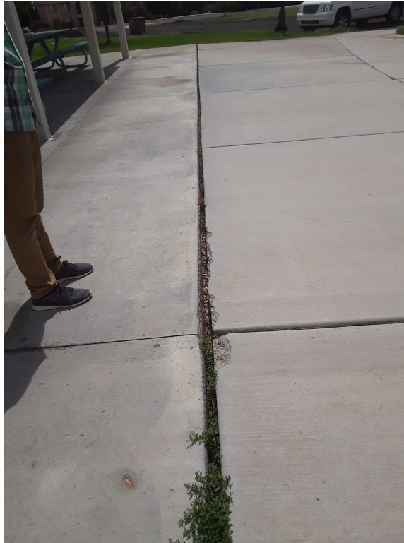
Figure 4. Damage Concrete Pad
