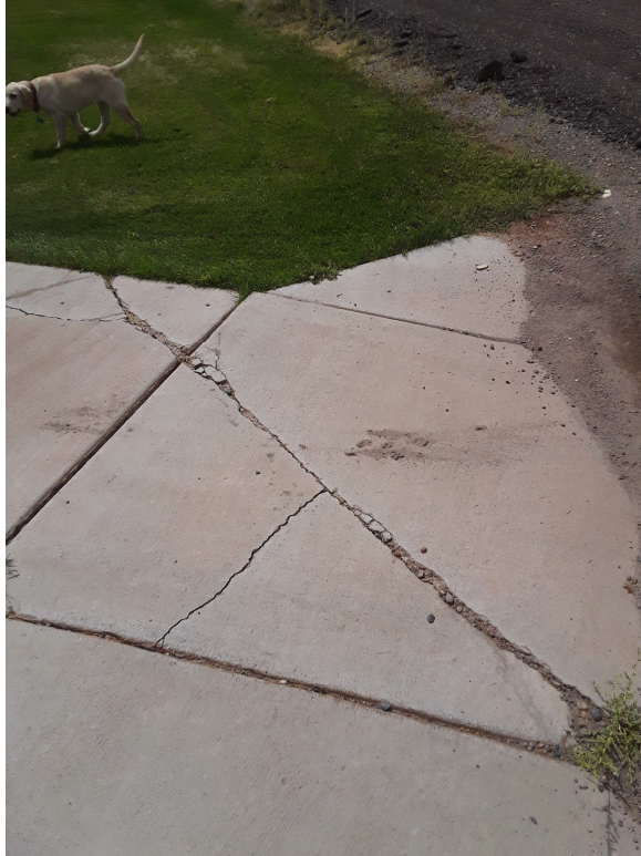
Figure 6. Damage Handicap Ramp
