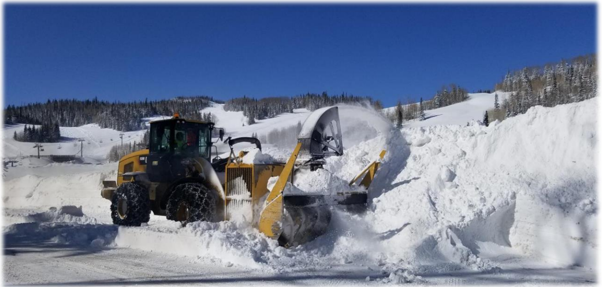
Blower running below Public Safety Building
