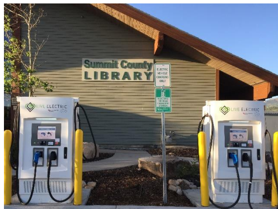
Figure 5. Summit County Library Electric Vehicle Charging Stations (photo provided by Summit County)
