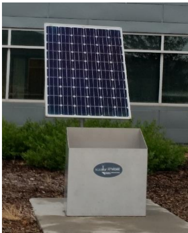
Figure 198. Solar PV Example at Summit County Health Department.
