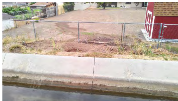
Cracking in the concrete liner causes water to seep into adjacent yards and properties.
