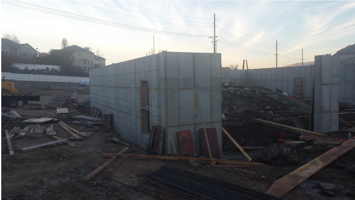
Figure 5- The small opening on the left wall is the personnel door into one of the two truck bays.
