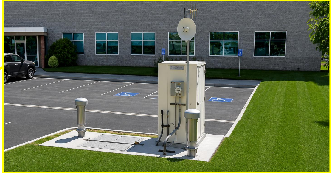
SSLC Meter Vault 2890 South 600 West
