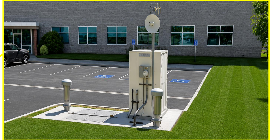
SSLC Meter Vault 2890 South 600 West
