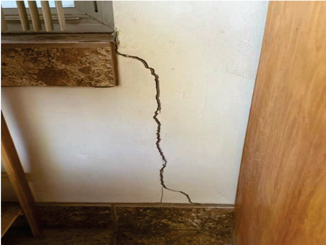
9. Existing Crack in West Wall of Kitchen
