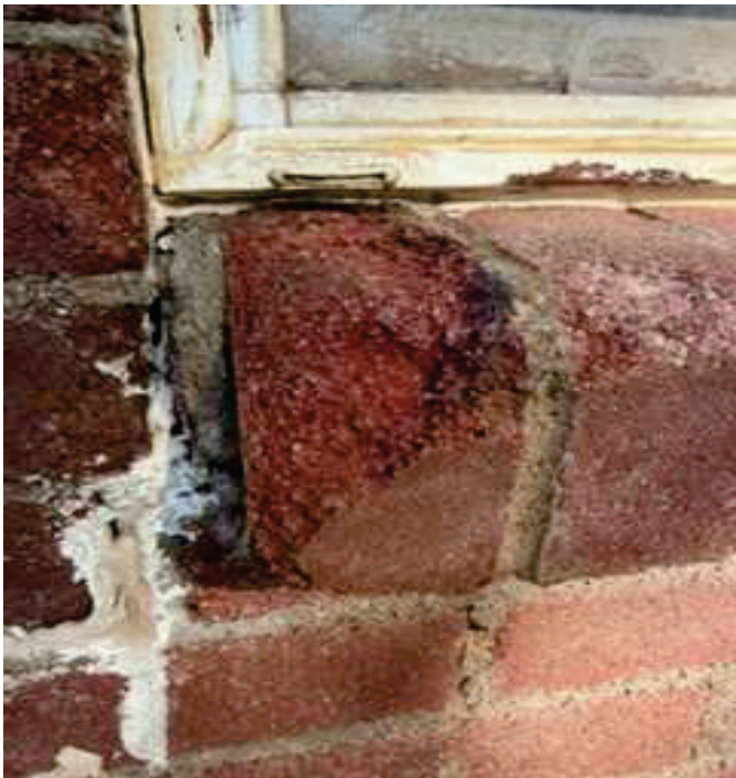
12. Existing Exterior Brick in Deteriorated Condition
