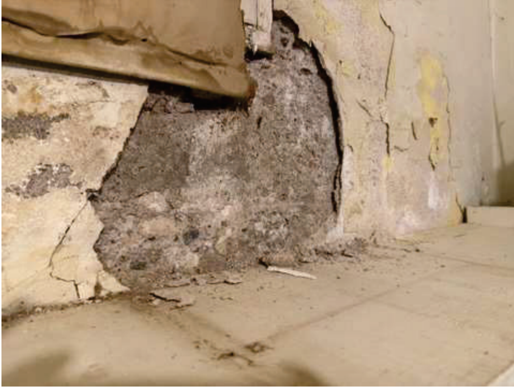
5. Existing Concrete Cracking & Spalling in Basement Wall
