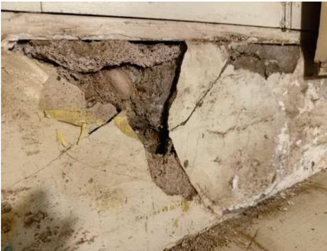
4. Existing Concrete Cracking & Spalling in Basement Wall
