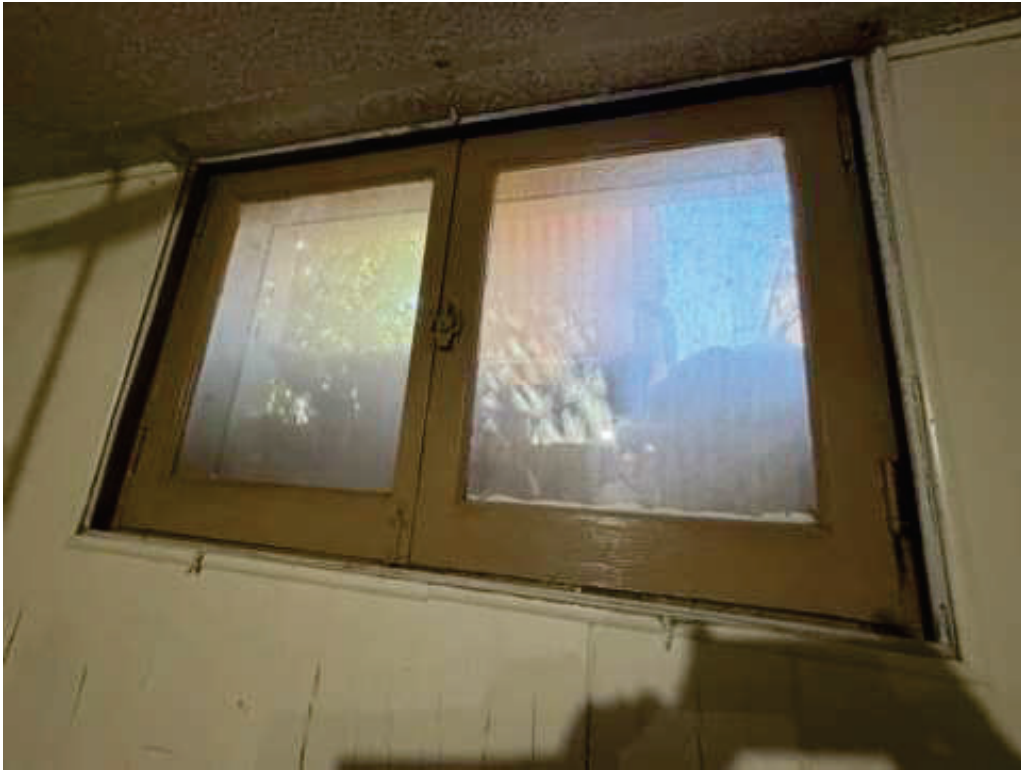
3. Existing Basement Window w/ Deteriorated Frame
