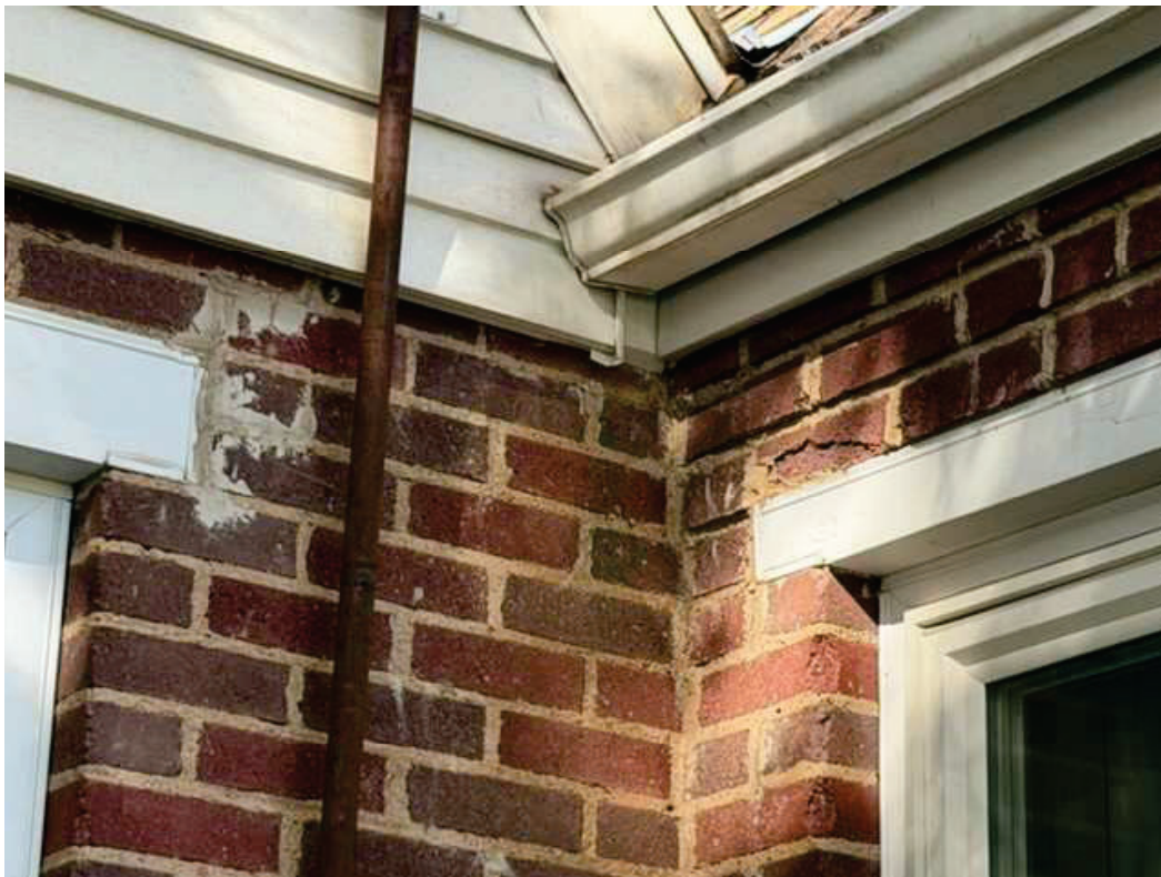
14. Existing Exterior Brick Displacement & Deterioration
