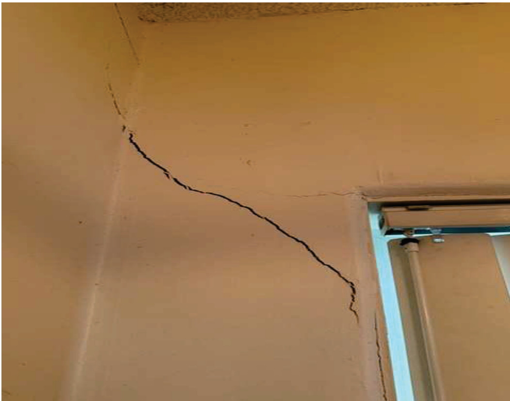
10. Existing Crack in West Wall of Entry
