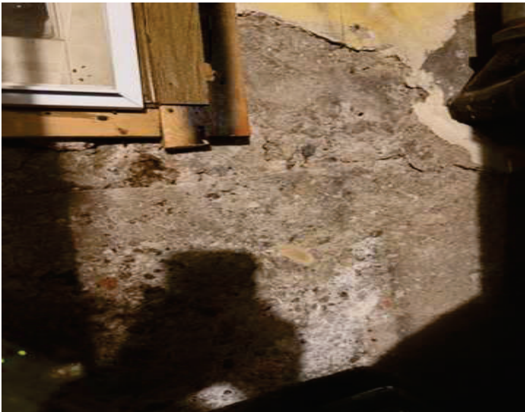
6. Existing Concrete Surface Spalling in Basement Wall
