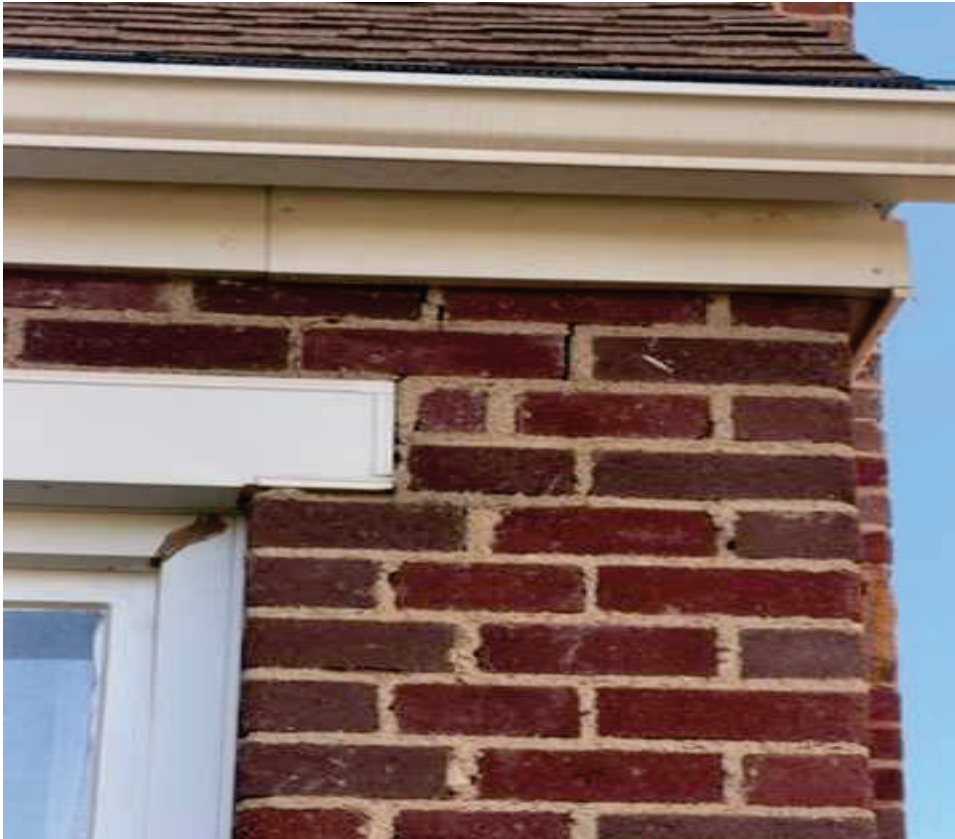
15. Existing Exterior Brick Joint Displacement
