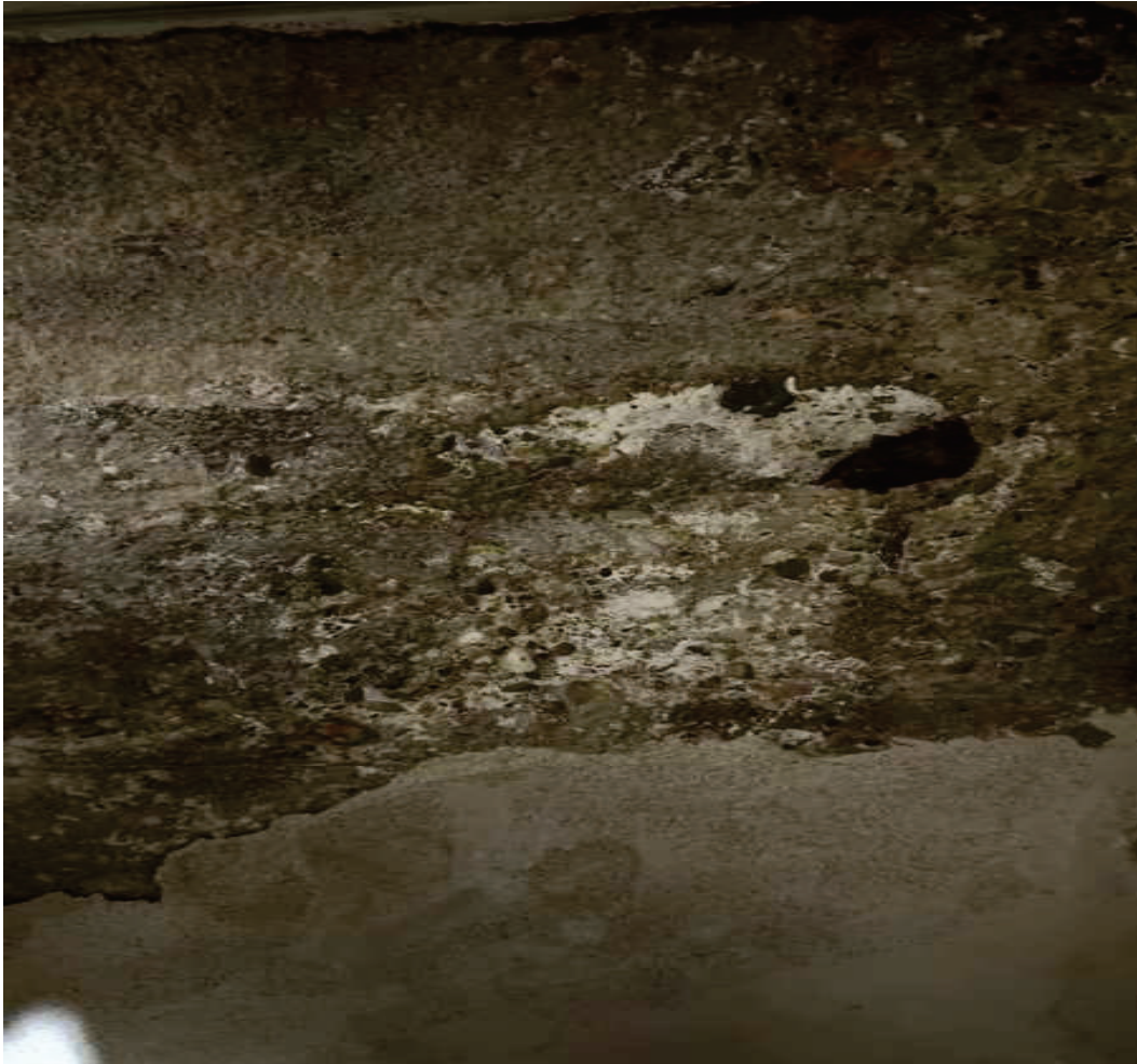
1. Existing Exposed Concrete Basement Wall – Surface Spalling
