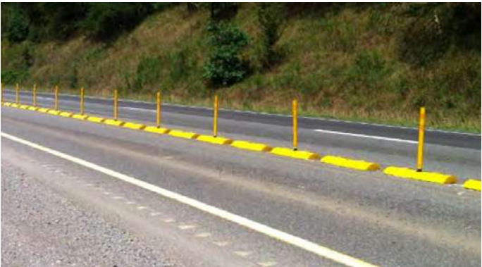
Flexible delineator with rubber curb
