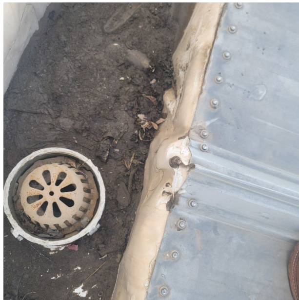
Figure 10 thru 14 - An improvised membrane gutter on the bottom edge of the galvanized metal roofing and inside the lower parapet wall has been a continuous problem.
