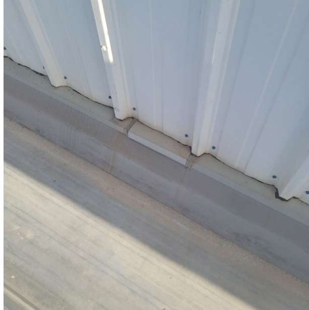
Figure 9 - Flashing on galvanized metal roof leaks in multiple locations.
