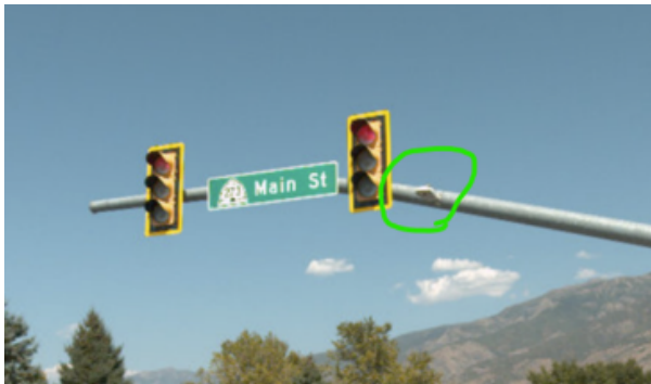
Figure 1: Under Mast Arm Light
