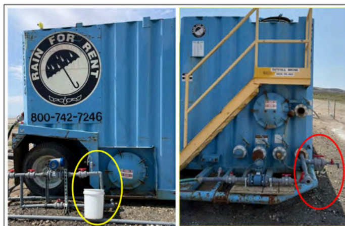
Figure 1. Samples were taken from the north tank for influent brine (valve circled in yellow) and the south tank for effluent (valve circled in red).
