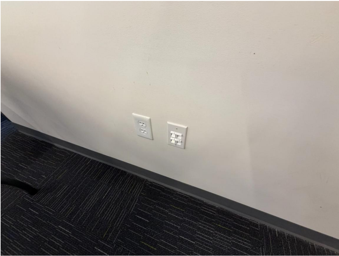
Figure 14. Police EOC - representative wall network connection.
