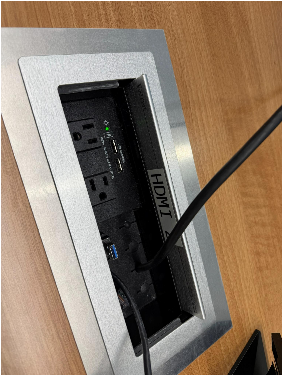
Figure 4. Staff Conference Room - table connection box (representative).
