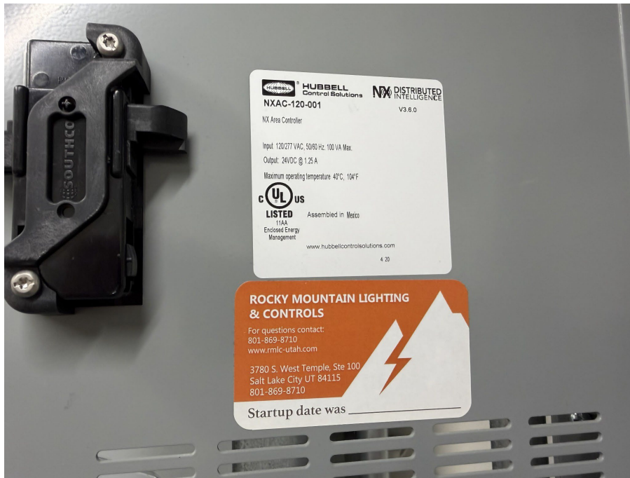
Existing Hubbell NX lighting control equipment - Photo 2
