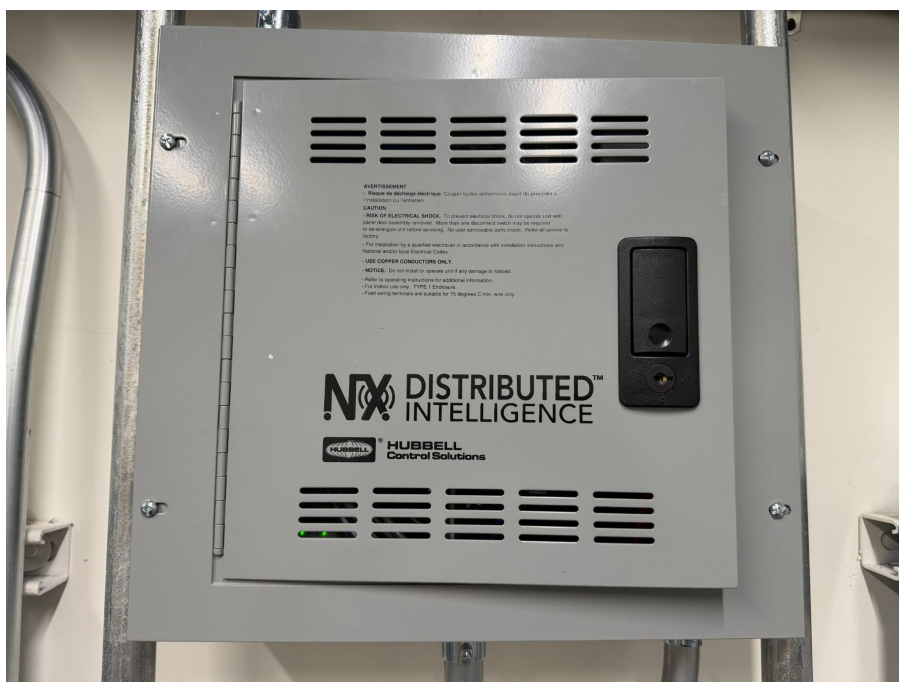
Existing Hubbell NX lighting control equipment - Photo 1
