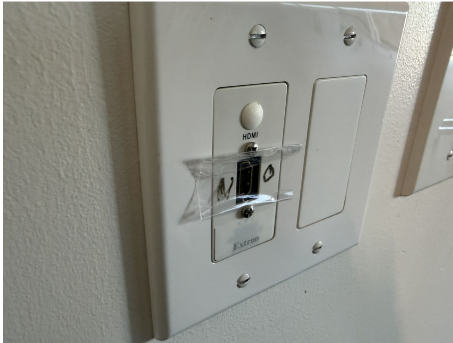
Existing Police EOC HDMI wall input – currently nonfunctional due to cut cabling.
