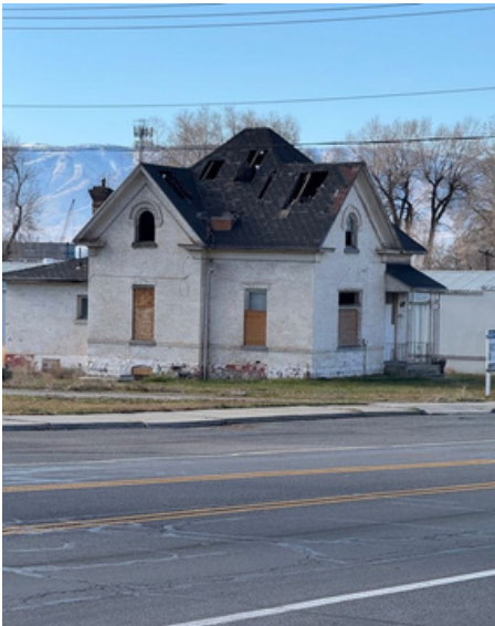
Example of dilapidated building in downtown
