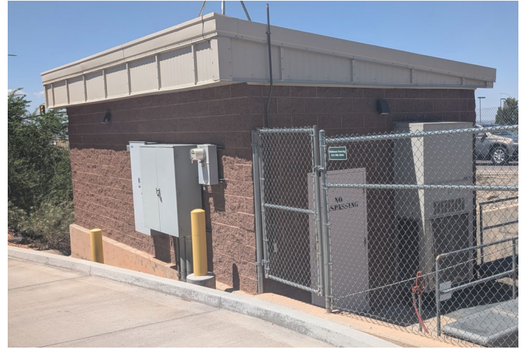
200 North Pump Station (built in 2008)
