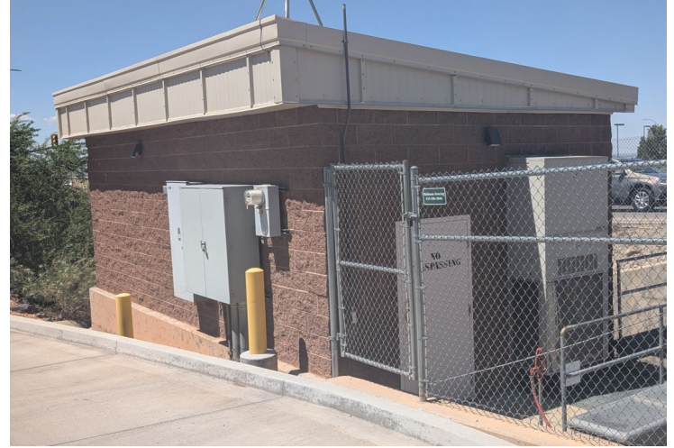
200 North Pump Station (built in 2008)
