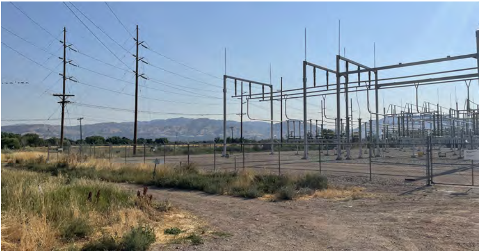
GROUND LEVEL VIEW OF RMP SUBSTATION WITHIN THE NATURA AREA.
