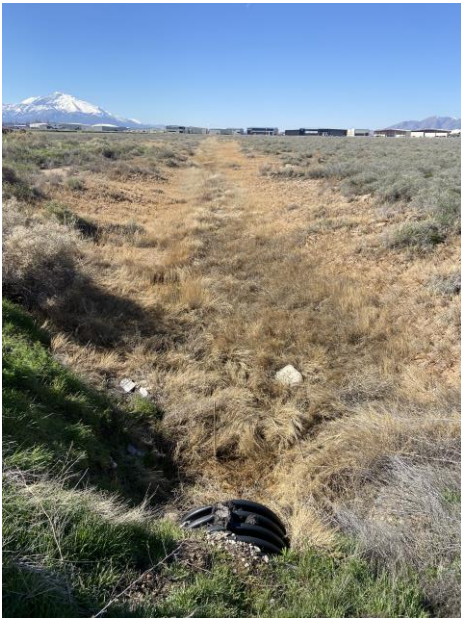
27-inch corrugated HDPE (Upstream side)
