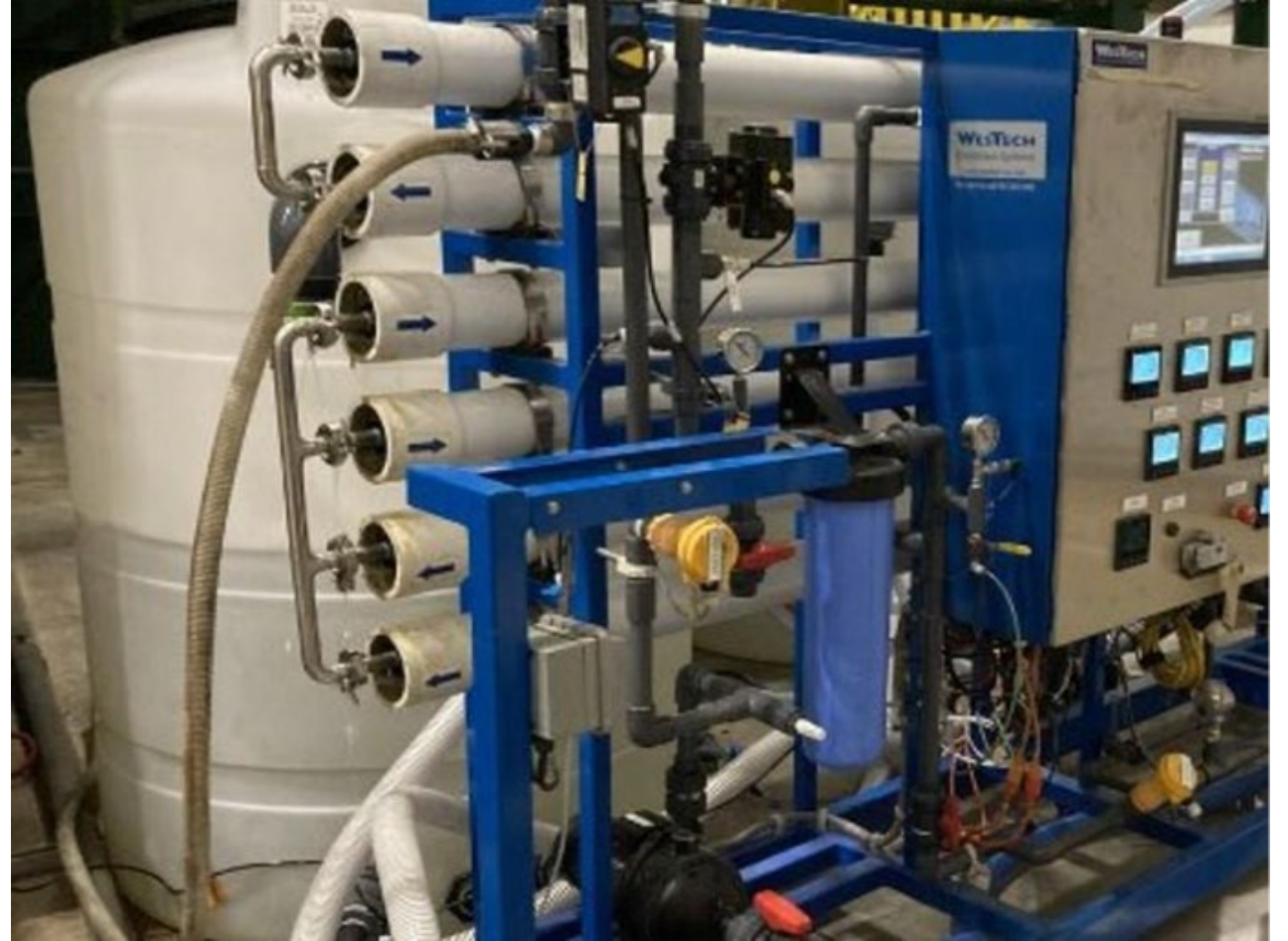
Reverse Osmosis Pilot Skid Canton, OH
