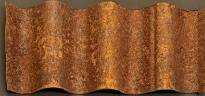
Rusted Metal Siding
