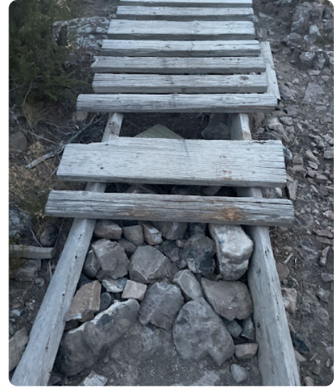
ObjID 37, Big Thunder: Bridge with missing planks.
