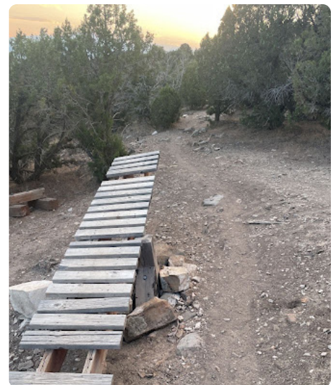
ObjID 47, Juniper: Feature with missing planks.
