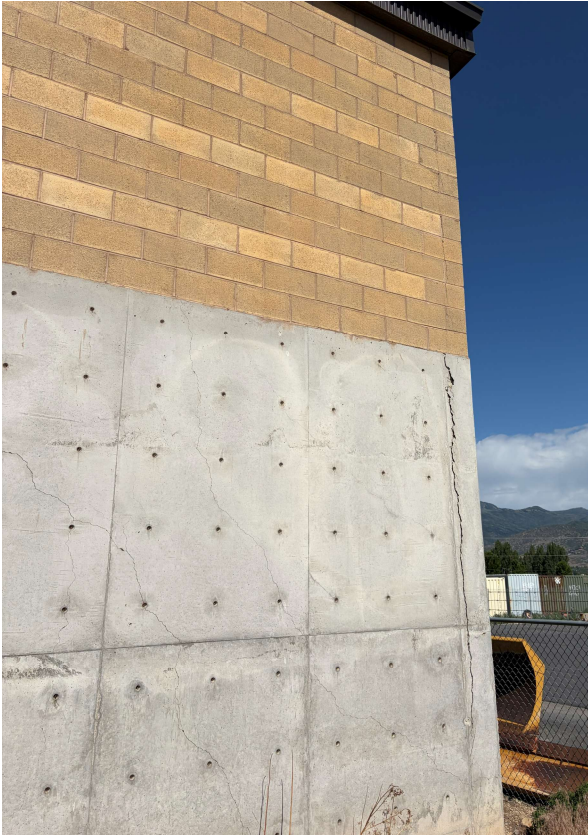
Figure 5: Diagonal cracking at east side wall
