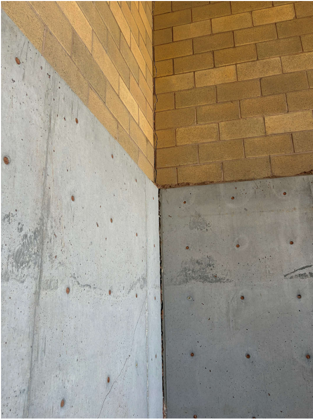
Figure 1: Interior north east corner cracking
