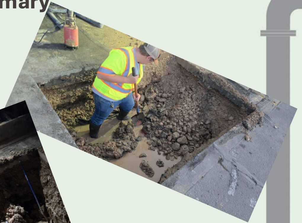
Water Leak on 700 S
