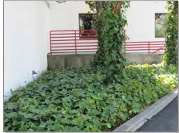
Figure 7: Downspout disconnected from parking lot
