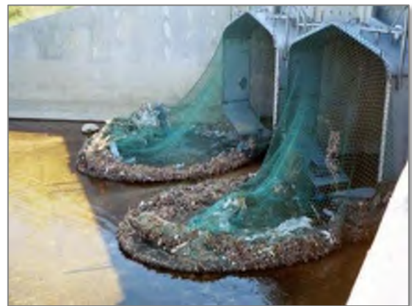
Figure 5: End-of-pipe trash netting
