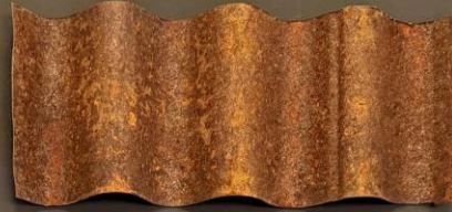
Rusted Metal Siding
