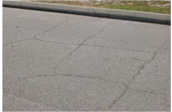
Figure 3 EXAMPLE OF BLOCK CRACKING
