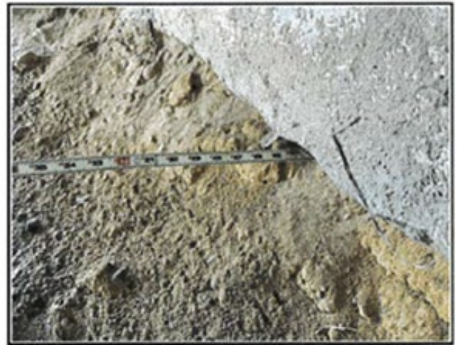
Abutment 1 Up to 24 IN Undermining
