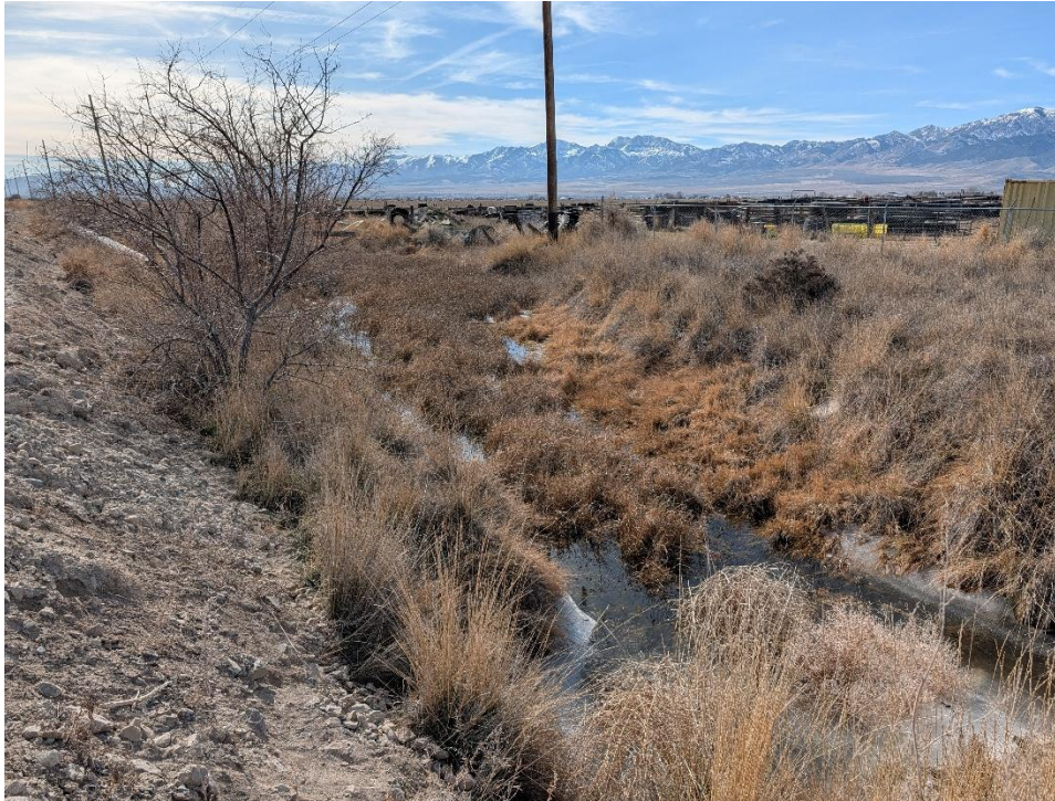
Figure 5-Surface water prior to culvert at Higley Road.
