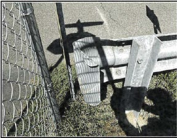
Railing 2 Distortion at South End
