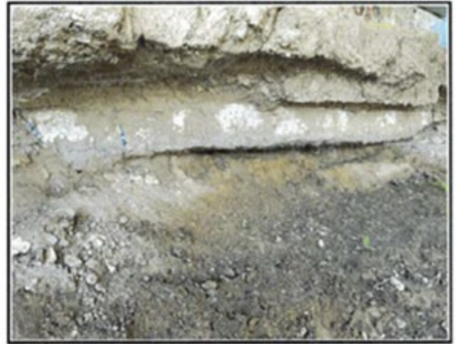
Abutment 1 Scour With Up to 20 IN Undermining
