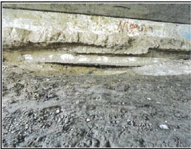
Abutment 1 Scour With Up to 20 IN Undermining
