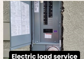
Electric load service center upgrade
