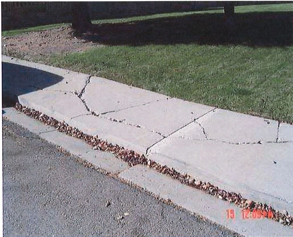
(Shown: Priority 1 – Cracking)
