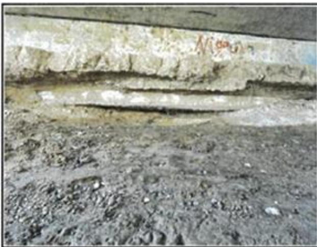
Abutment 1 Scour With Up to 20 IN Undermining
