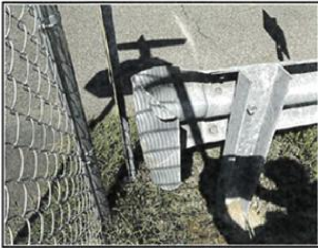
Railing 2 Distortion at South End
