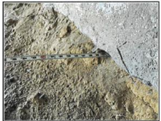
Abutment 1 Up to 24 IN Undermining
