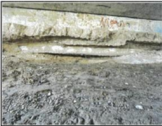
Abutment 1 Scour With Up to 20 IN Undermining
