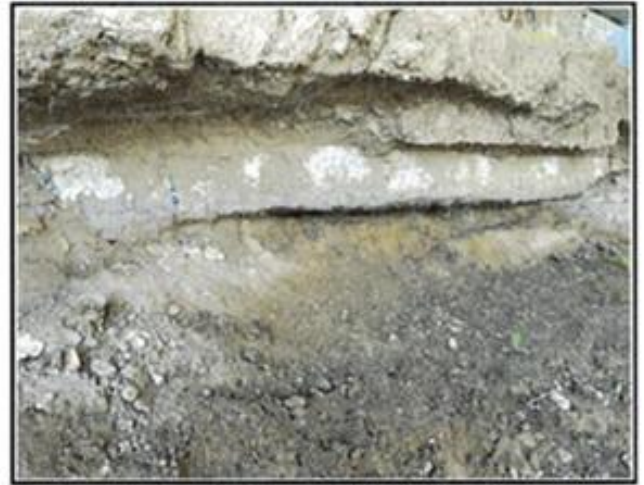
Abutment 1 Scour With Up to 20 IN Undermining
