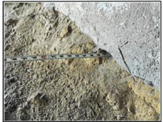
Abutment 1 Up to 24 IN Undermining
