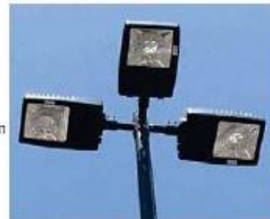
PARKING LOT LIGHT:
