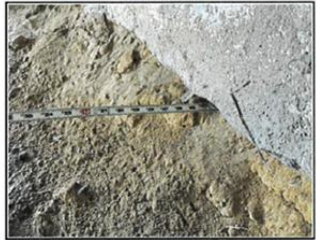
Abutment 1 Up to 24 IN Undermining
