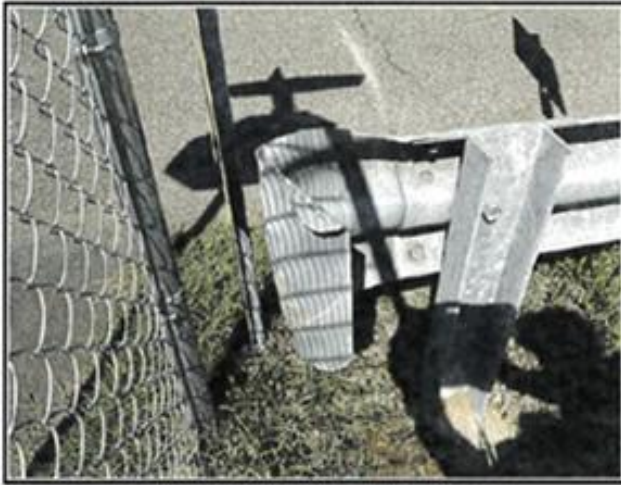
Railing 2 Distortion at South End
