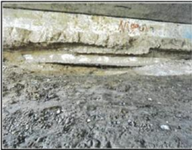
Abutment 1 Scour With Up to 20 IN Undermining
