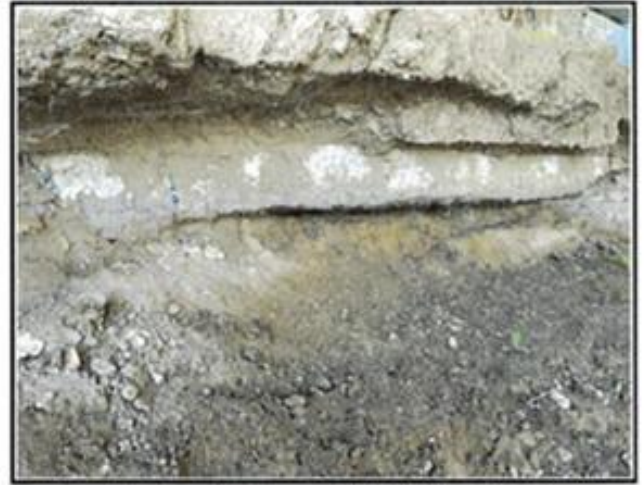
Abutment 1 Scour With Up to 20 IN Undermining
