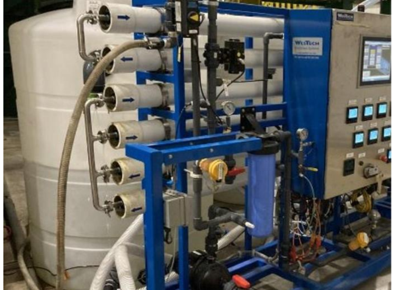
Reverse Osmosis Pilot Skid Canton, OH
